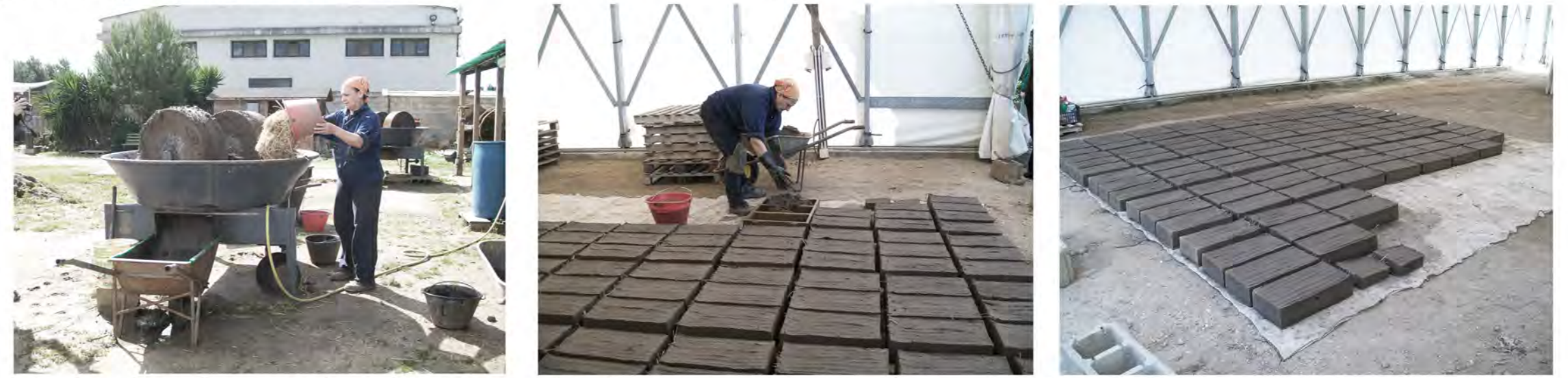
The local production of mud bricks sundried, a mixture of clay, silt, sand and straw (10x20x40 cm)
